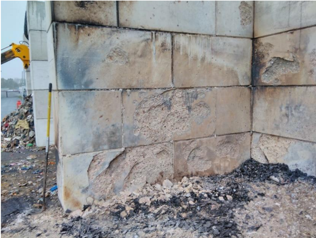
Figure 186: Fire Damage to block work wall
