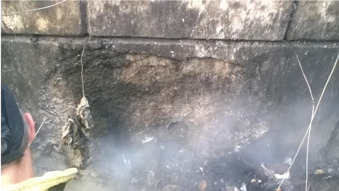
Figure 185: Damage to the concrete (post fire)
