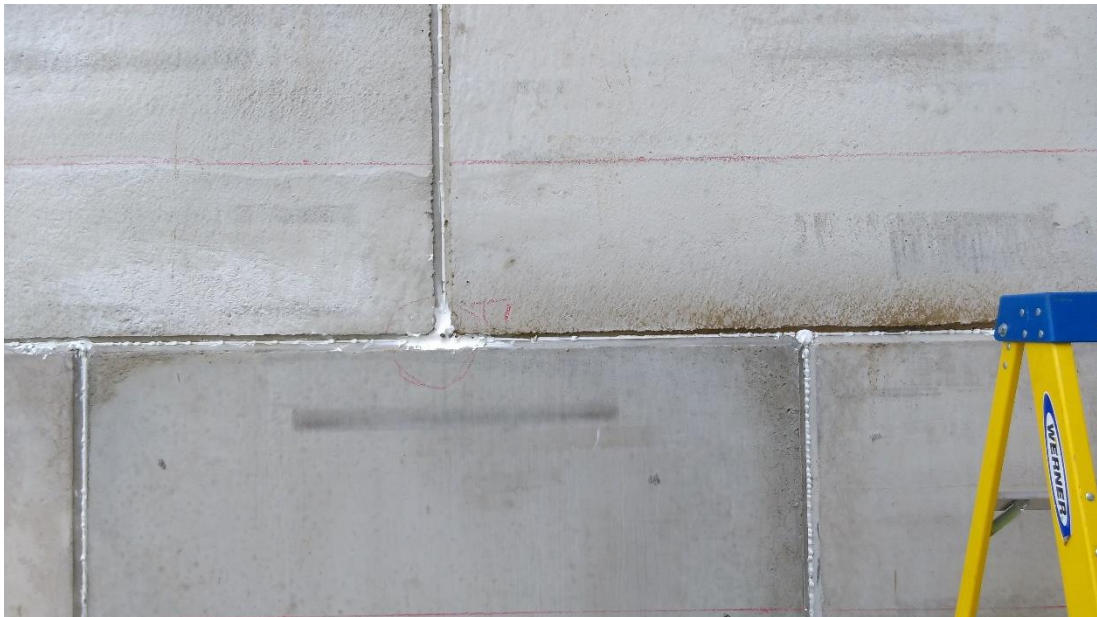
Figure 179 Intumescent mastic used to seal joints in one elevation
