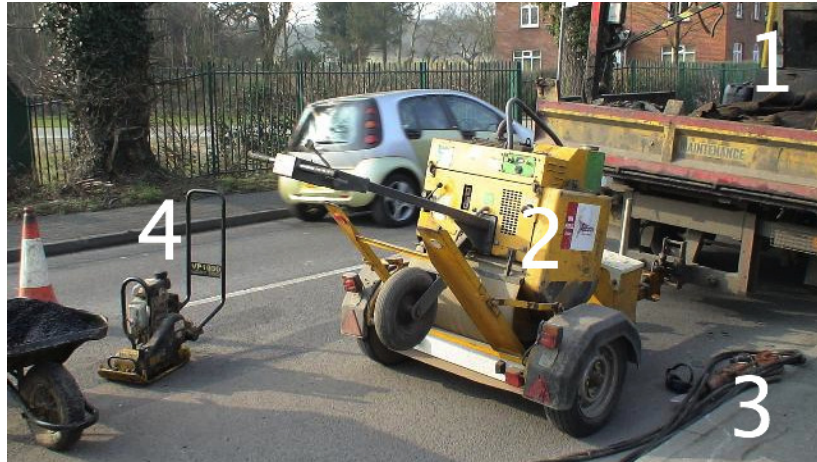
Fig. 1. Key Equipment Used for Road Patching: 1 – Van, 2 – Petrol Powered Drum Roller/Air Compressor (Stored on Trailer), 3 – Air-powered Pavement Breaker, 4 – Petrol Powered ‘Wacker’ Plate Compactor.
