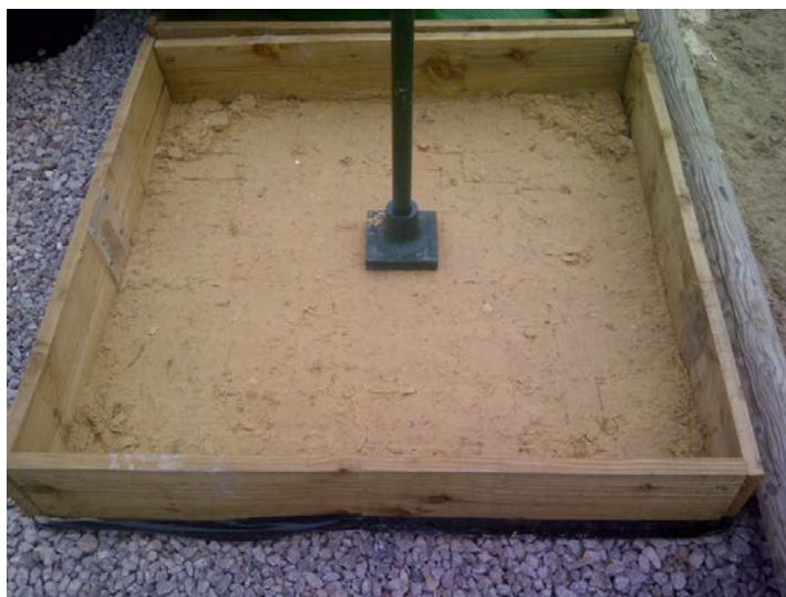
Plate 2.1.3 The “elephant foot tamper” being used to compact the first layer of sand.
